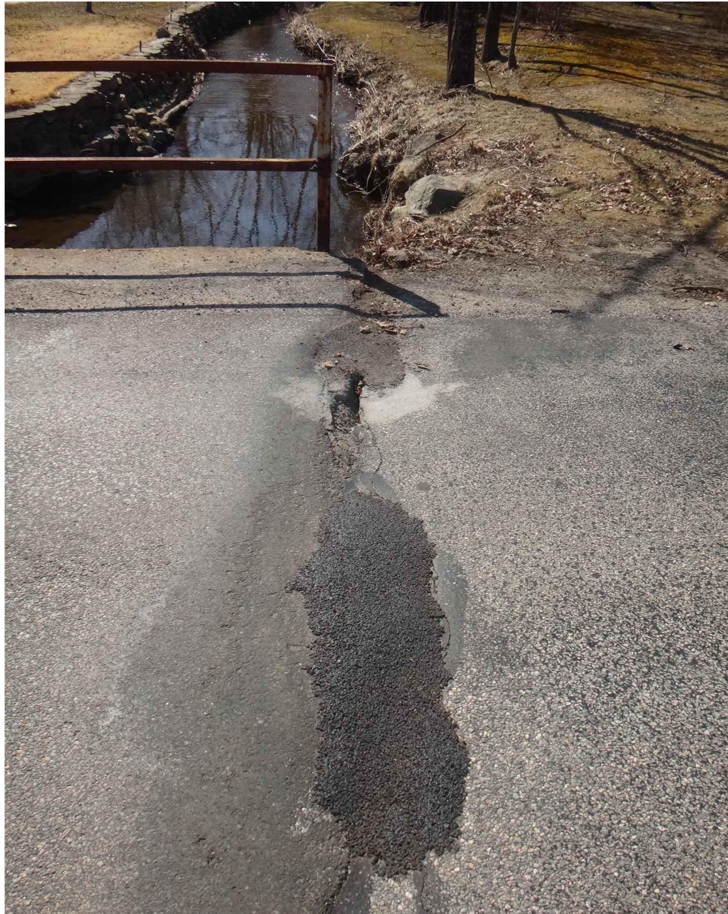
West Abutment joint at the south end with patches, settlement and a void, looking south.
