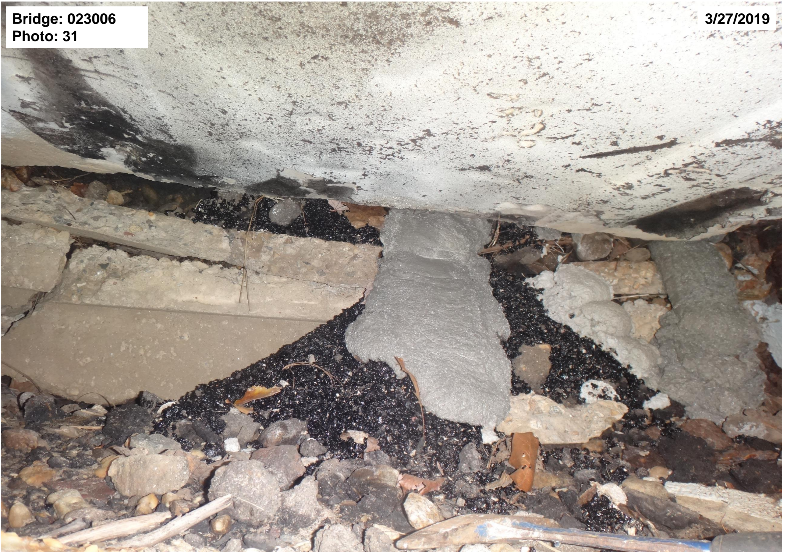
West Abutment backwall in Bay 6 with severe deterioration, settlement and bituminous patch material, looking west.
